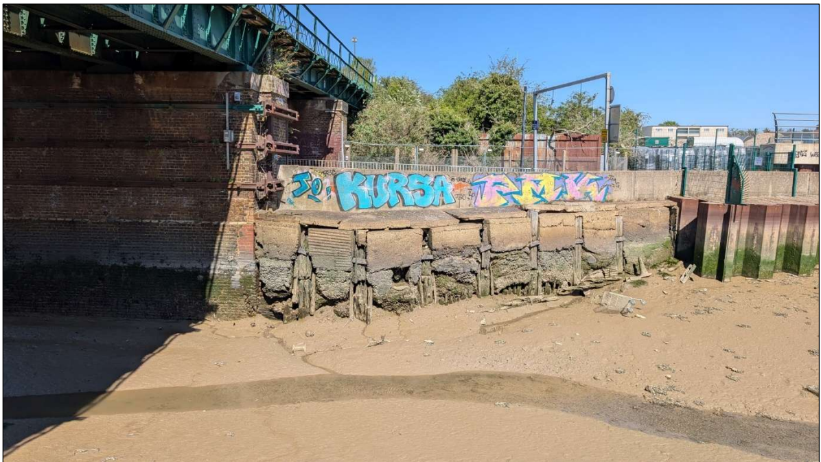
Figure 2-5 Flood defences at SNF15.
